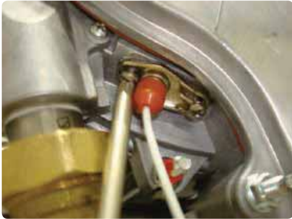
Figure 137 Removal of Ignition electrode
