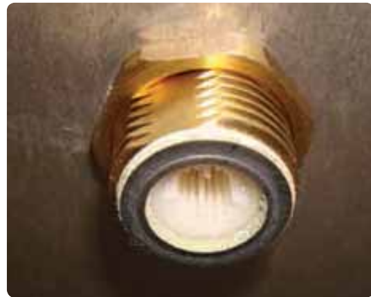
Figure 43 DHW inlet has a filter screen
